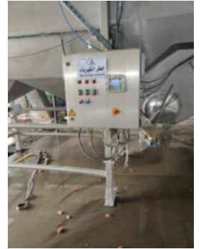
one electrical panel was Not provided by rubber mat in the Production hall.jpg
